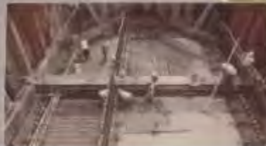
Concrete slabs and steel provide structural stability to support the pump station's long life.
