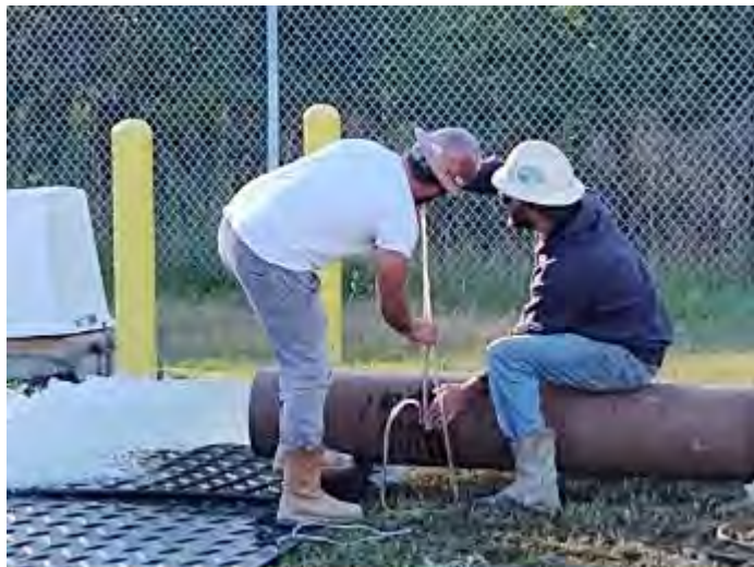
NP_MAR_01 pumping 2,800 gpm during testing
