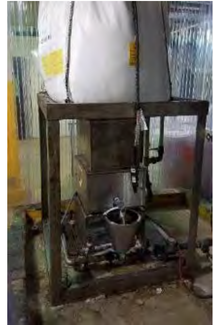
New Polymer skid to provide greater reliability
