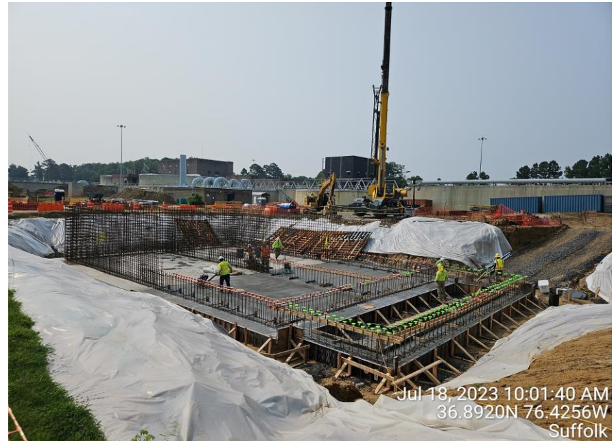
Medium Voltage Switchgear Building
