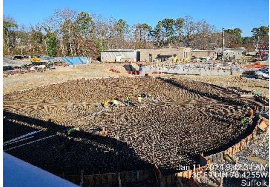
Primary Clarifier No. 5
