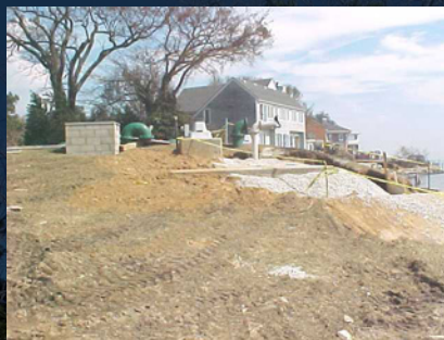
Inset: Hurricane damage to the Claremont Avenue Pump Station (left) and rebuilding of the pump station property (right).
