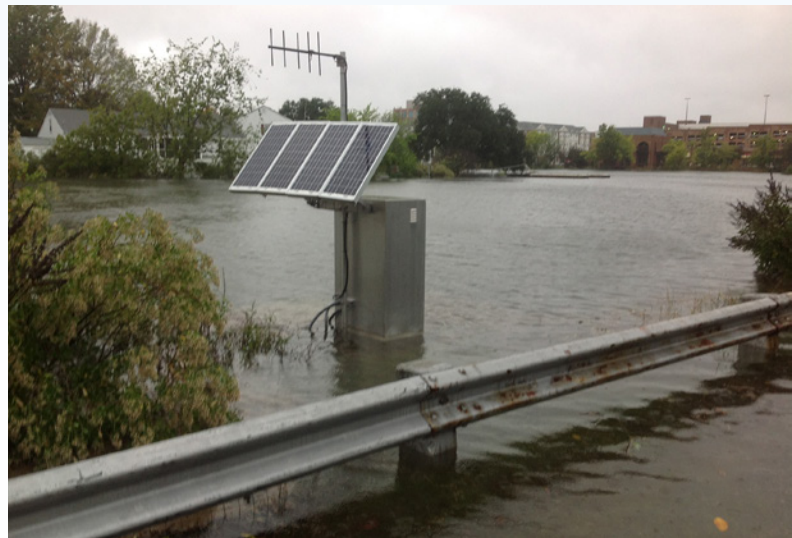
Flooding along Bridge Street at the Tidegate Vault.
