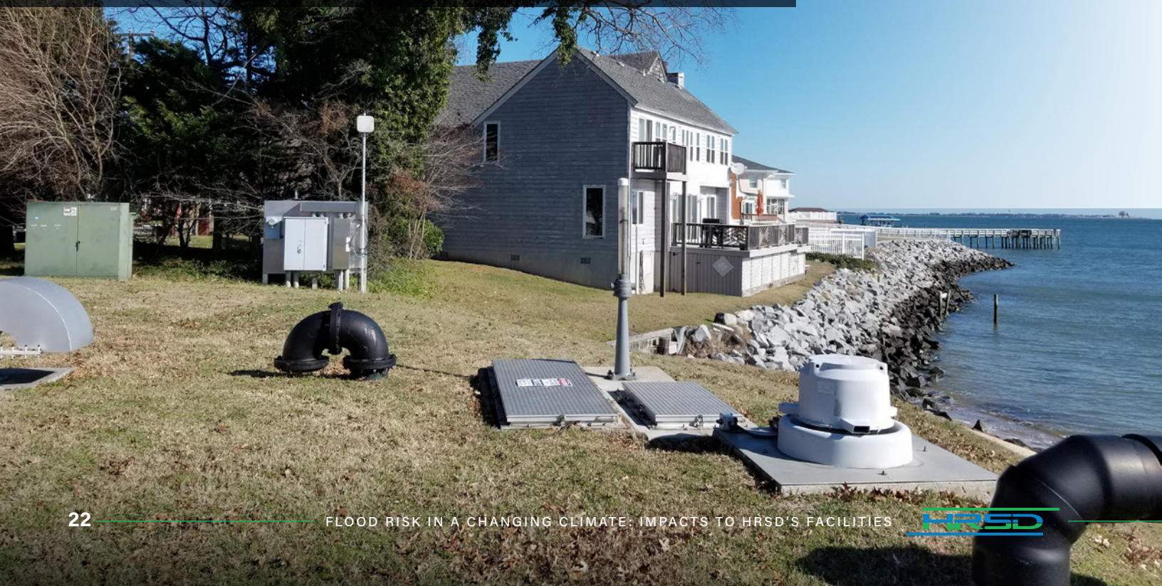
Below: Claremont Avenue Pump Station (underground) adjacent to a residences.
