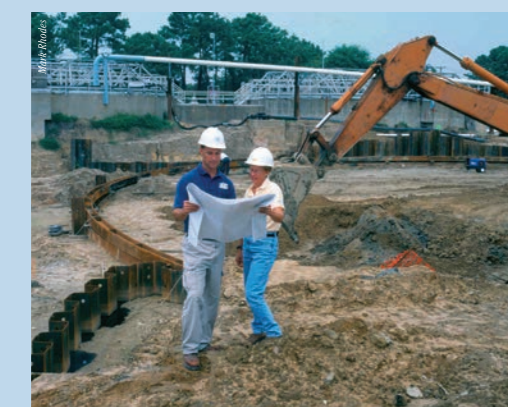
Project Manager Bruce Husselbeck and Karen Harz, HRSD's first female plant manager, review plans for the Chesapeake-Elizabeth Treatment Plant upgrade that began in 2004.
