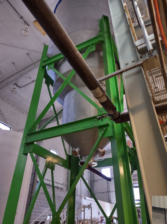
↑ New P2K reactor
