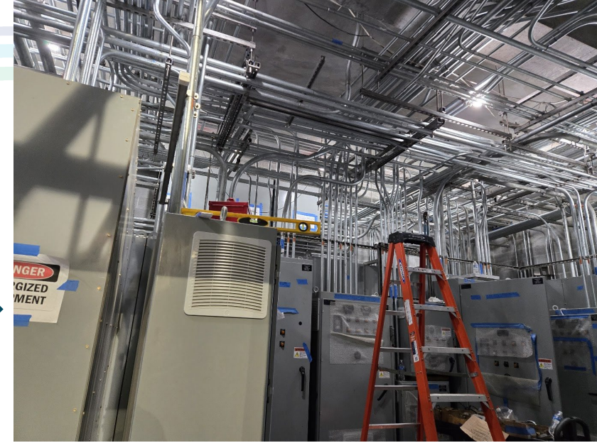
New Electrical Room
