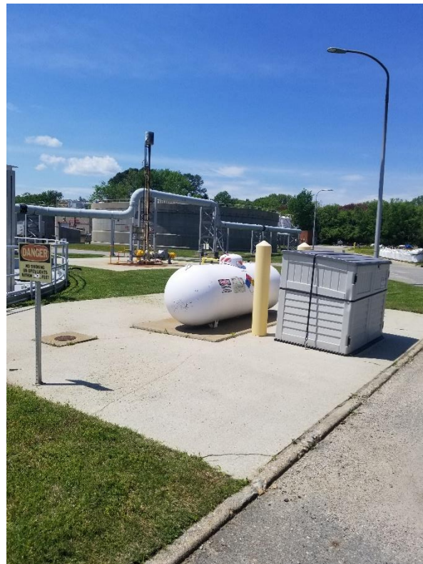
Propane tank and spill kit storage container at JRTP facility.
