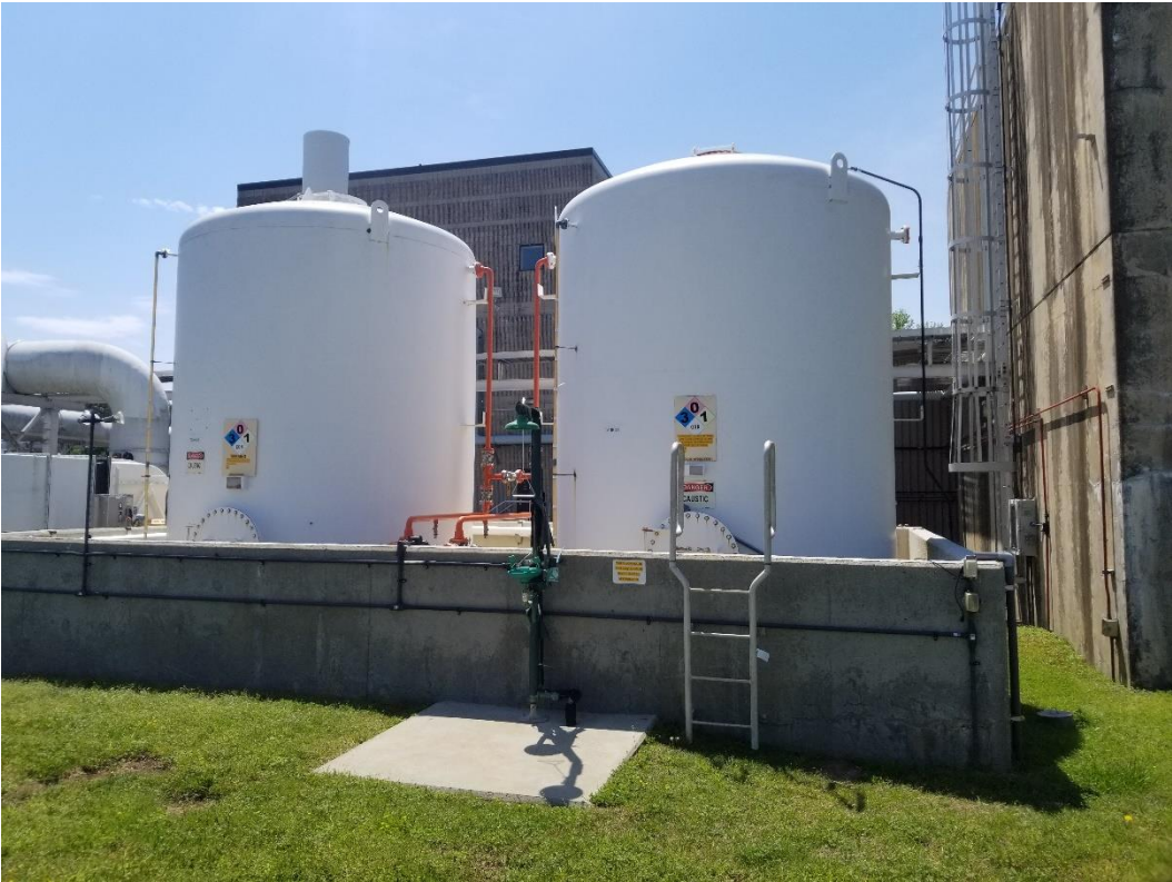
Sodium hydroxide ASTs and associated containment area at JRTP facility.
