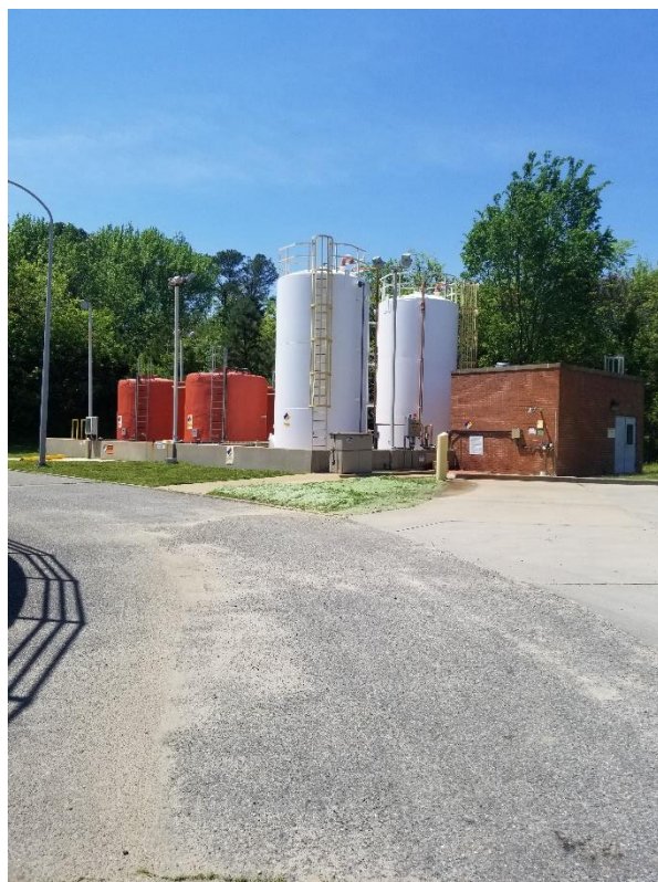
Sodium hydroxide and ferric sulfate ASTs and associated containment area and phosphorous removal facility at JRTP facility.
