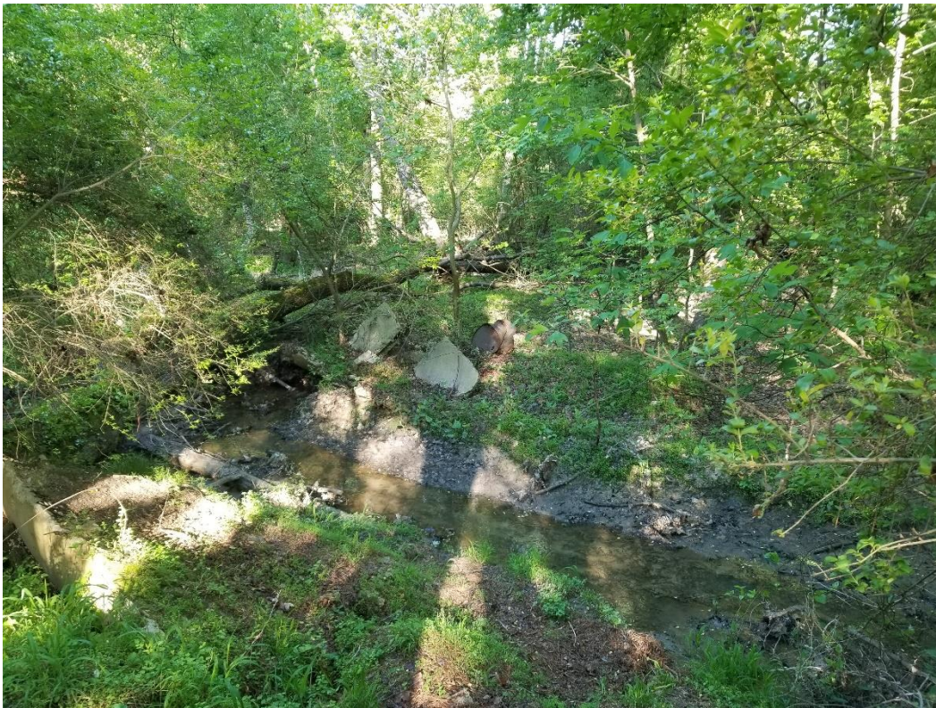
Debris at base of slope northwest of the JRTP sites as viewed from opposite slope.
