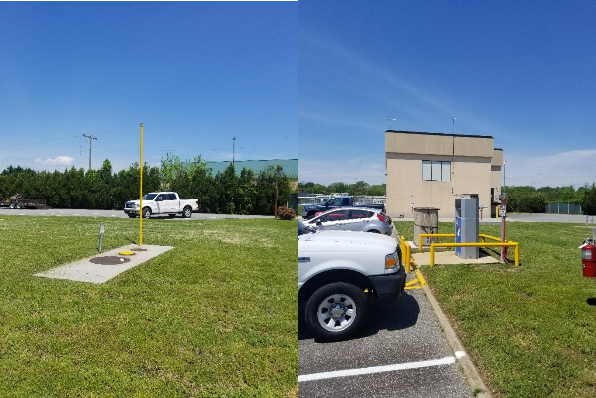
Vent pipe, fill port, fuel dispenser, and spill kit storage container for gasoline UST at JRTP facility.
