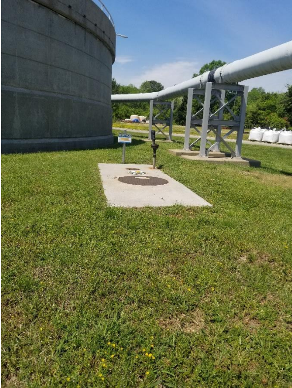
No. 2 fuel oil UST fill port and vent pipe at JRTP facility.
