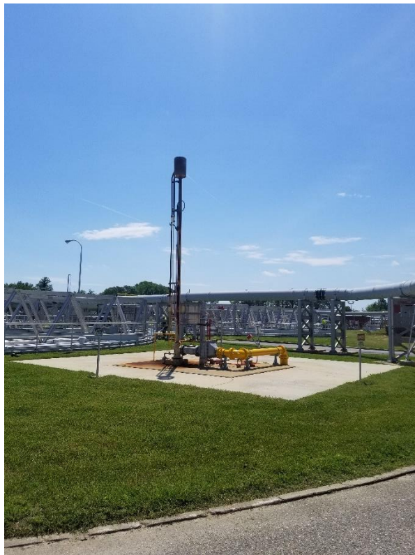
Methane flare and associated piping at JRTP facility.
