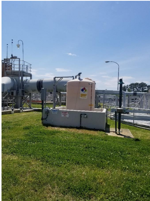
Muriatic acid AST and associated containment area at JRTP facility.
