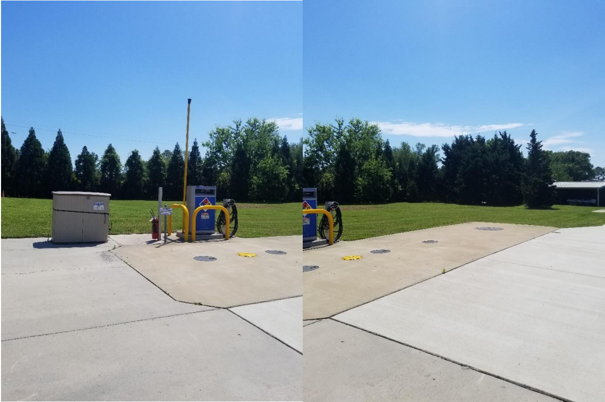
Fuel pump, fill ports, vent pipe, and spill kit storage container for diesel fuel UST at JRTP facility.
